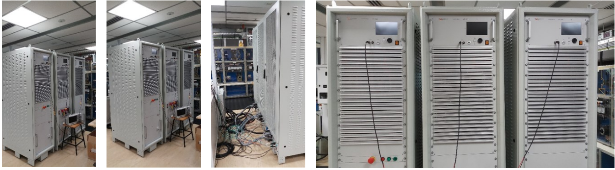
Fig 4.14: The three-phase 45kVA power amplifier that acts as an interface between OPAL-RT and the physical microgrid testbed in Clean Energy Research Laboratory in NTU.
